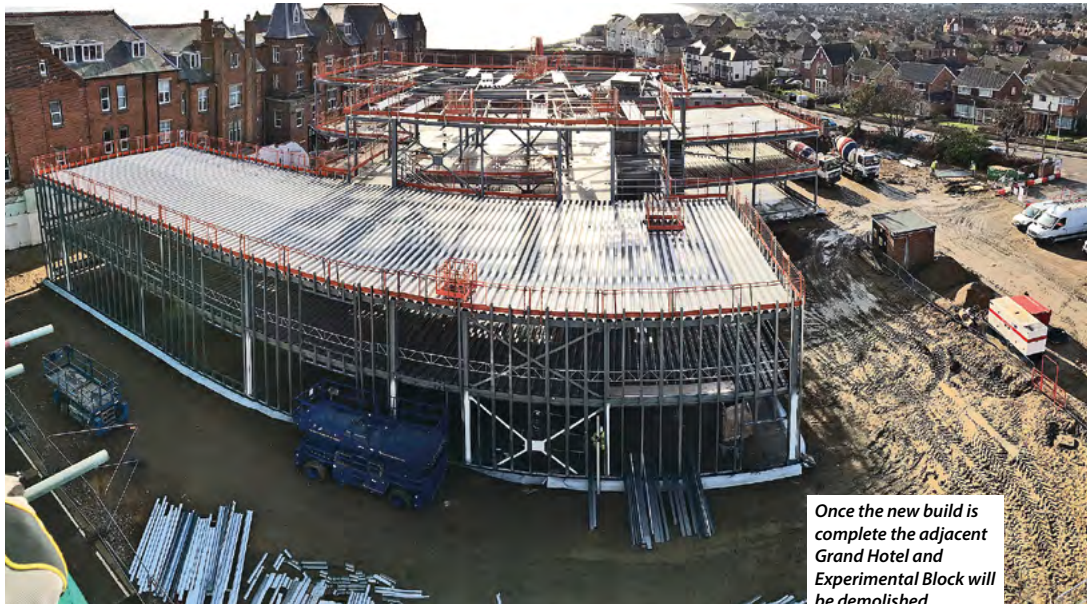
All of the steelwork will be left exposed within the new building
