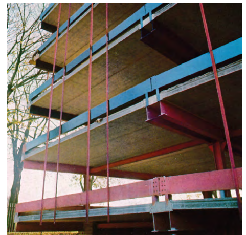
Steel work before final painting. The light vertical members are for panel fixings
