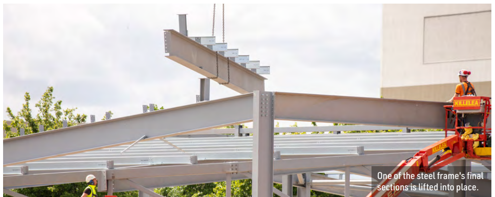
Two mobile cranes were used by James Killelea to install the roof rafters.
