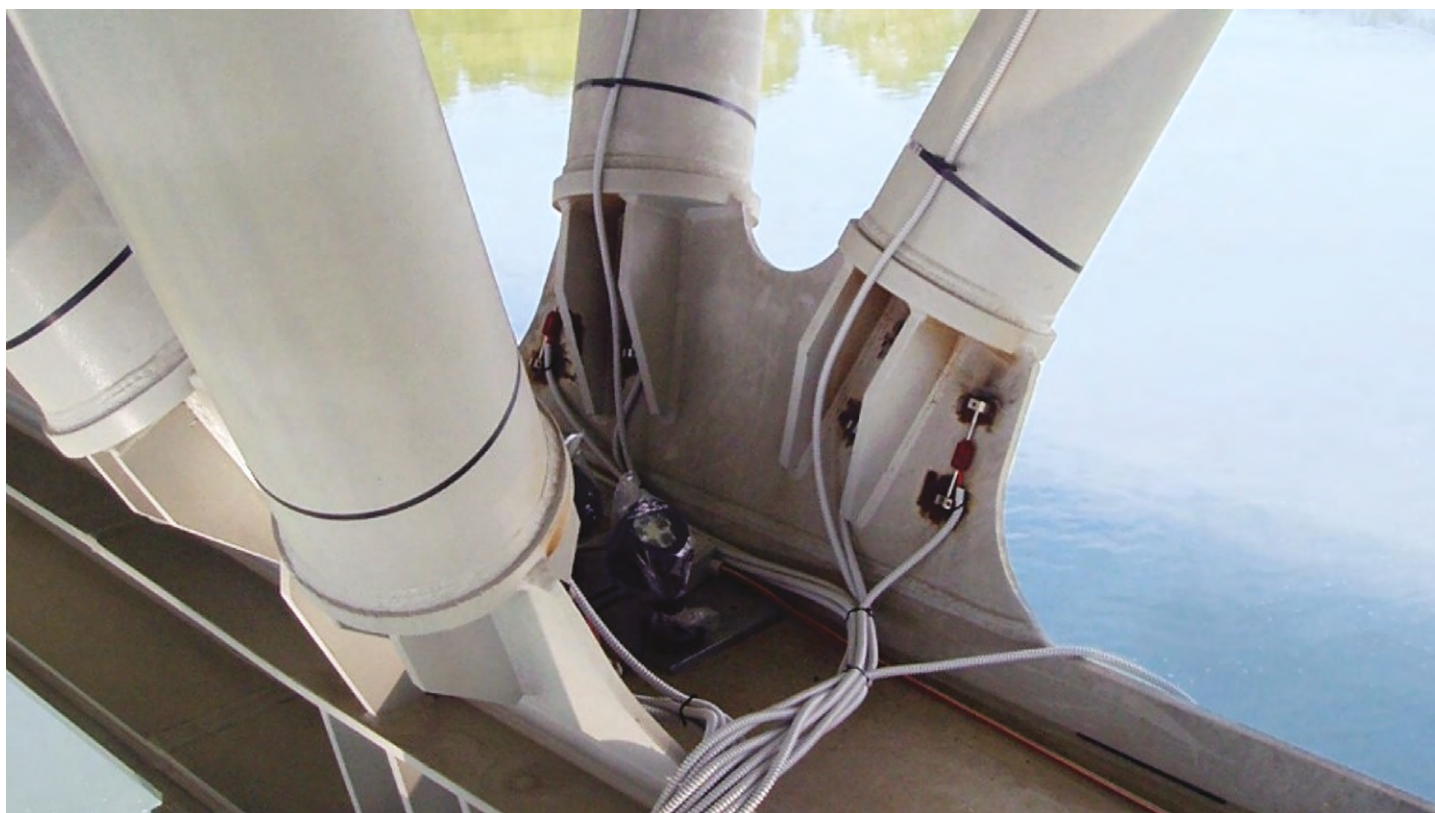
Figure 2: Vibrating wire strain gauges installed on steelwork (courtesy Sisgeo.com)
