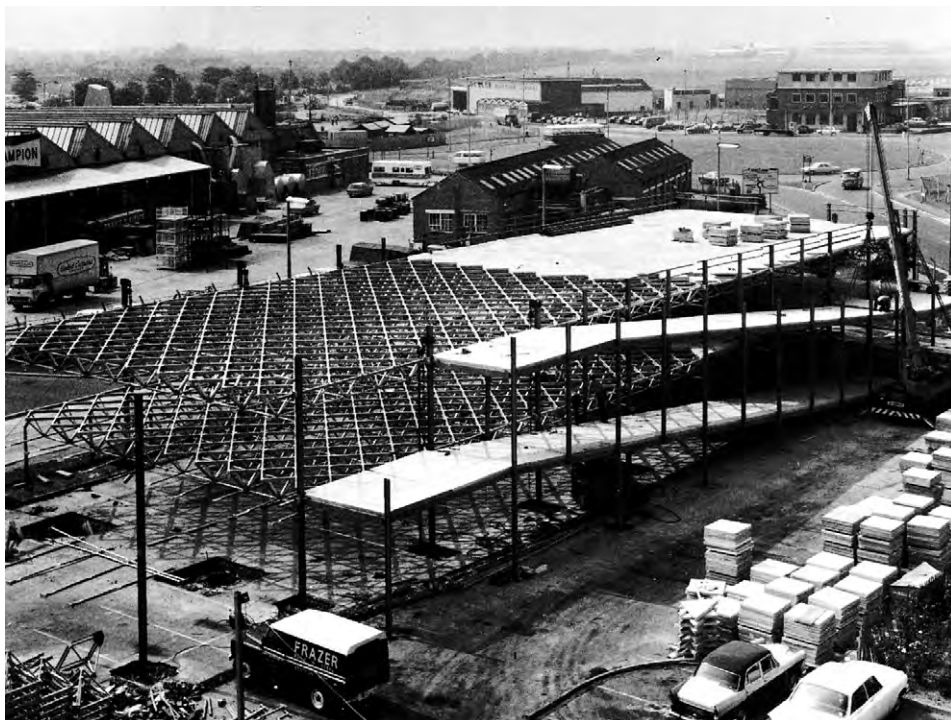
This view of the car-park during construction shows the structural system and diagonal grid form. Decks were assembled on the ground and lifted in one piece.
