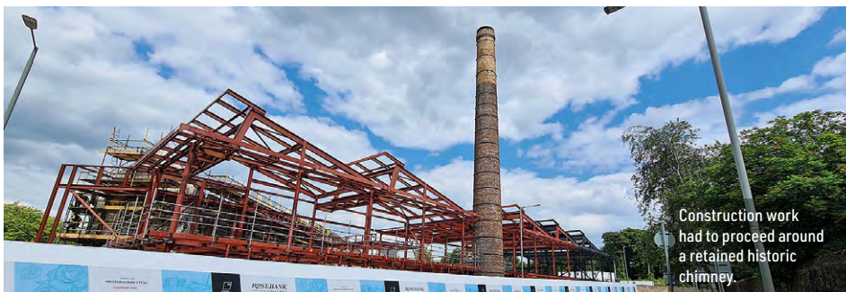
Steel erection was complicated by the tight and confined footprint of the site.
